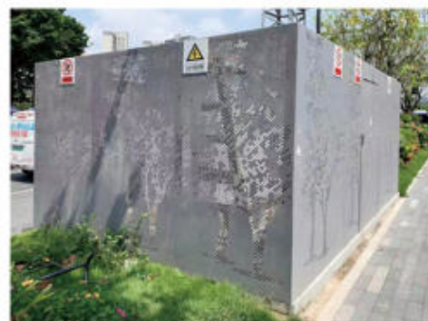
● 深圳龙华城中村变电站围栏 Shenzhen Longhua Chengzhong Village Substation Fence
